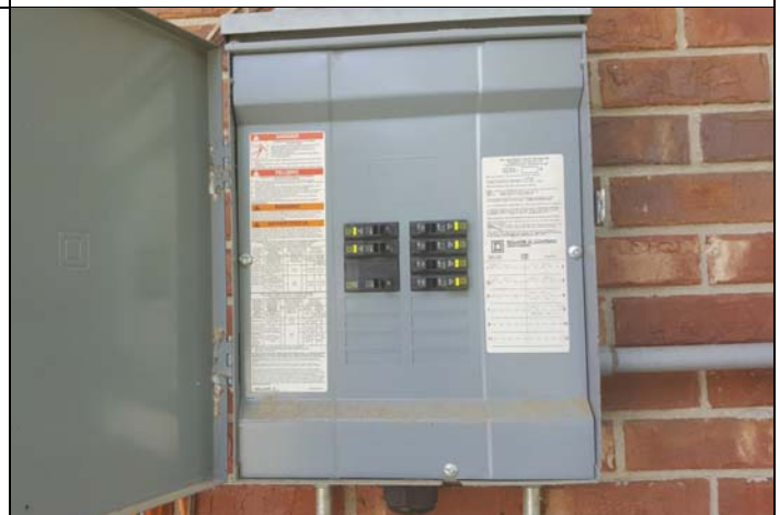
18. Distribution panels are provided as needed throughout the facility.
