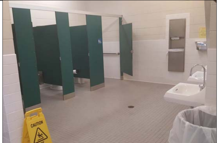
14. Each building has multi-user toilet rooms.
