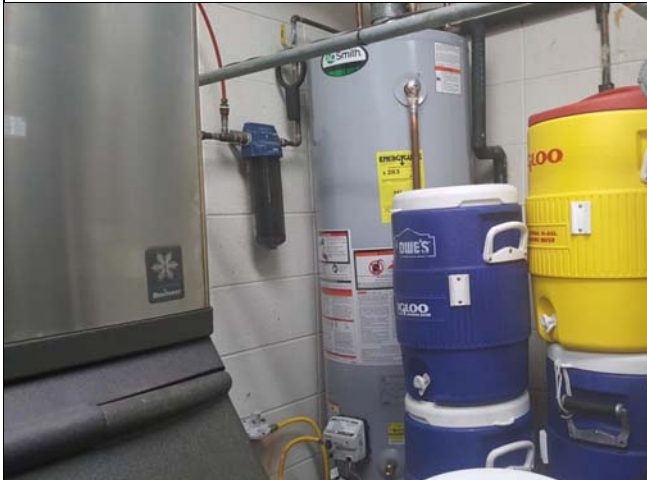
15. A gas-fired domestic water heater serves each of the buildings.
