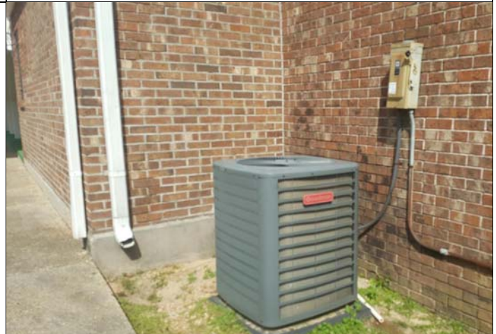
16. Both buildings are heated and cooled by split systems.
