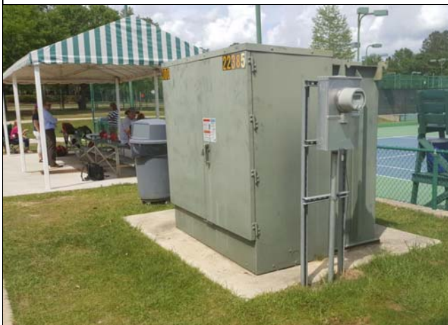
17. A transformer and meter is provided on the east side of the east building.
