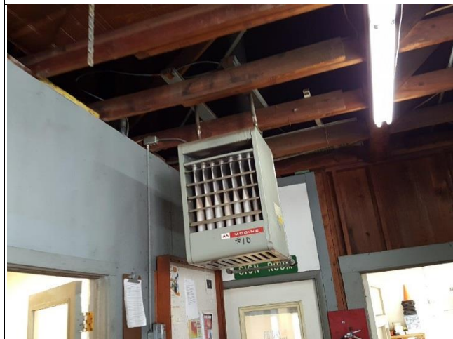
15. Heating at the Sign Shop and Vehicle Warehouse buildings is provided by ceiling hung heaters.
