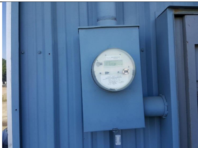
16. The main service panel disconnect switch and meter are located at the southwest corner of the Office building.
