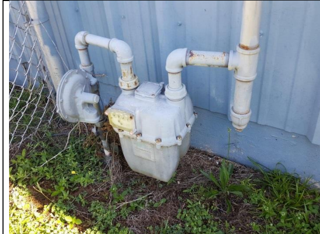
13. Incoming main gas service/meter is located at the south side of the Office building.
