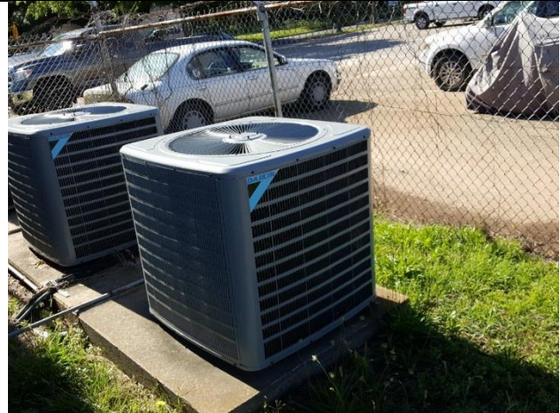
14. Air conditioning and heating at the Office building is provided by split-systems with condensers located on the south side of the building.
