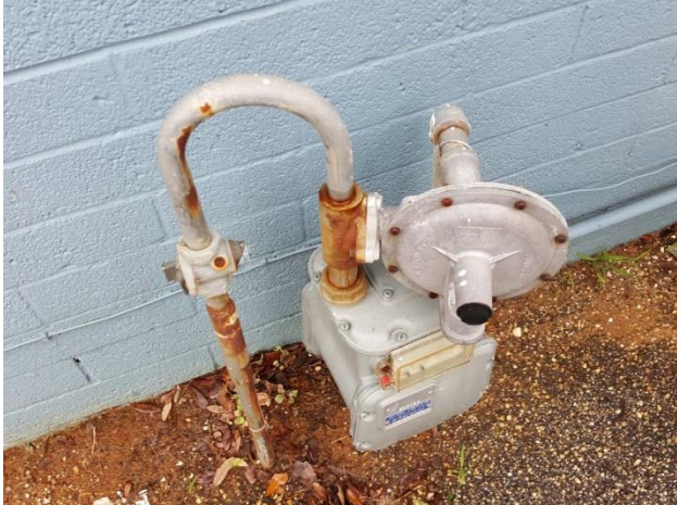
13. Independent natural gas lines and meter are provided at each building.
