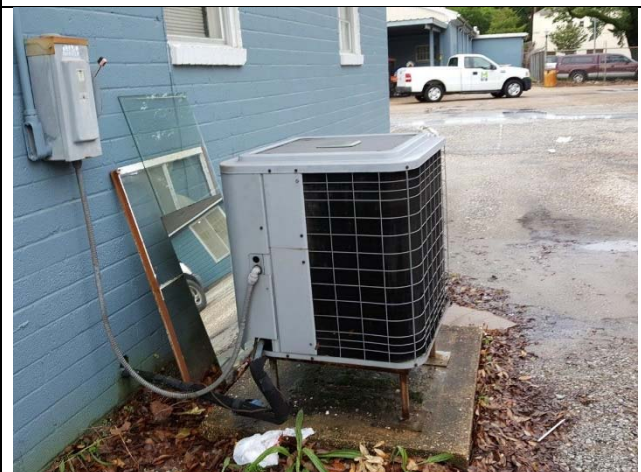
17. Condensers are located outside the building.
