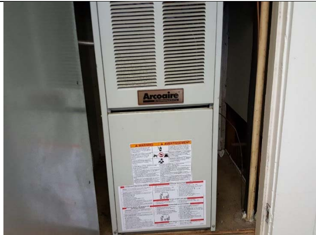
16. Air conditioning is provided by split systems with AHU's located inside the building.
