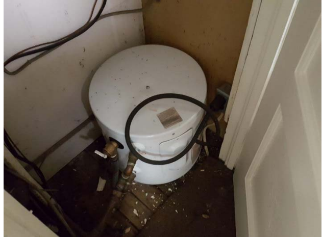
14. Domestic hot water at the Landscaping Services building is generated by an electric resistance DWH.
