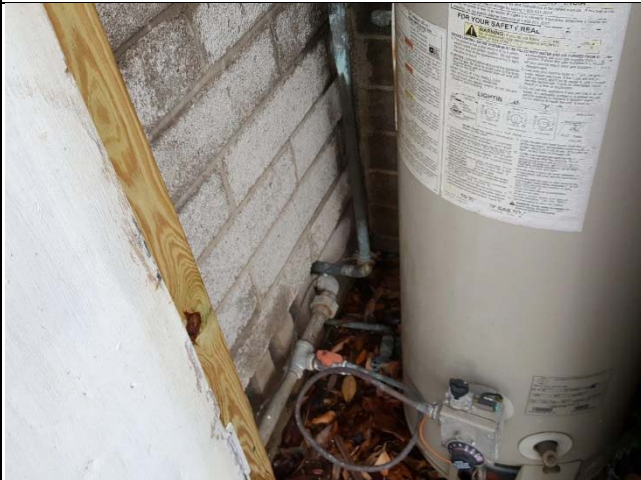
15. Domestic hot water at the Eastern Maintenance Building is generated by a gas-fired DWH.
