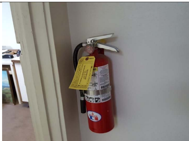
18. Fire protection is provided by wall mounted fire extinguishers.
