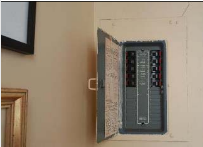
17. Distribution panels are mounted throughout the facility.
