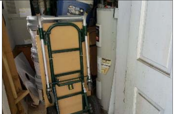
14. Hot water is provided by a 30-gallon Bradford White electrical resistance DWH located in a mechanical/ storage room.
