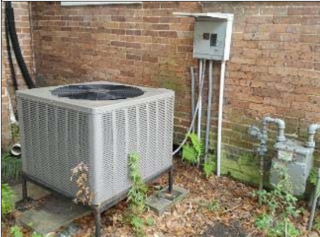
15. The building is heated and cooled by split systems with condensers and a package unit located on the west side of the building.
