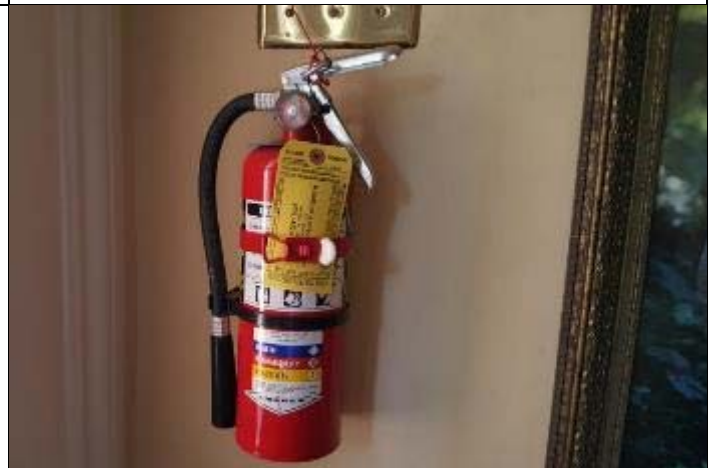
18. Wall mounted fire extinguishers are provided throughout the building.
