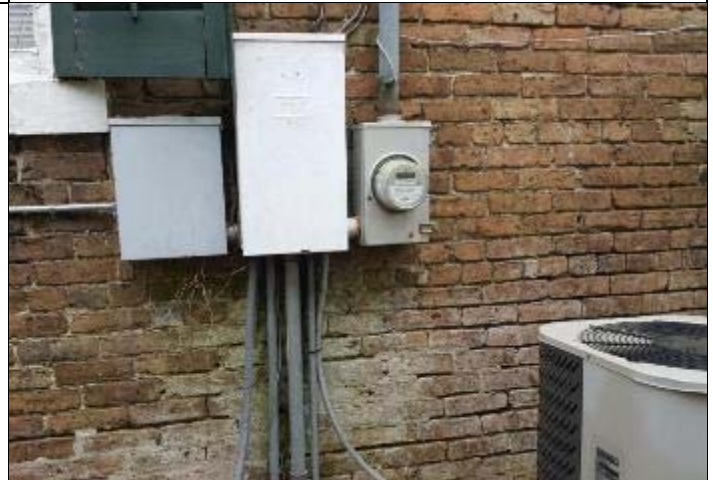
16. The main electrical service enters the Subject from a pole mounted transformer on the west side of the building to exterior switchgear.
